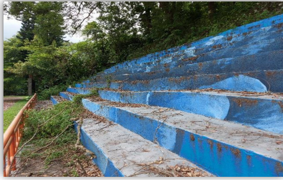
Fig.3 Deformation of play ground stairs
