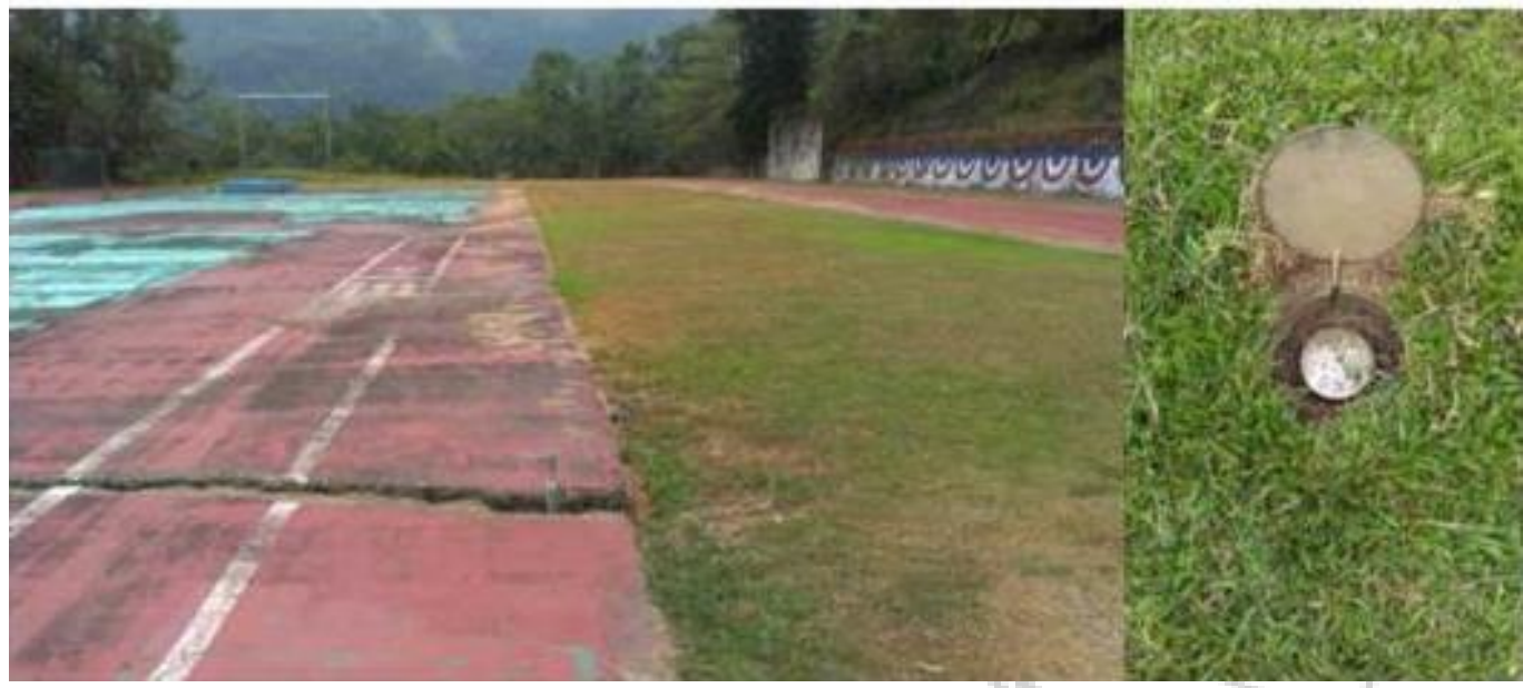
Fig.4 Fractures on play ground runways and leveling point G416
